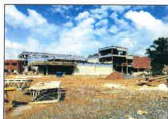
Construction continues at the student and faculty entrance of the elementary school being built at 123 N. Gramby St. What will the new school be called? The school is taking suggestions at manheimcentral.org . Photo by Rochelle Shank
